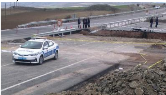
Figure 23. Fatal accident caused by underpass/culvert construction (Int. res. 3).
