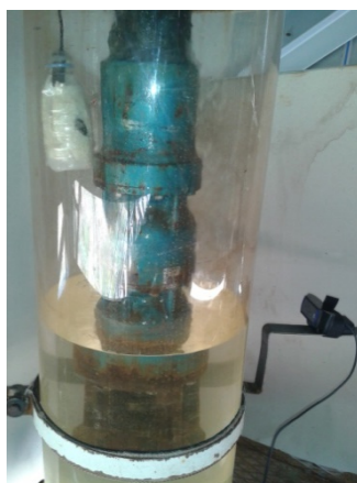
Figure 3. Submersible pump and connection of the camera
