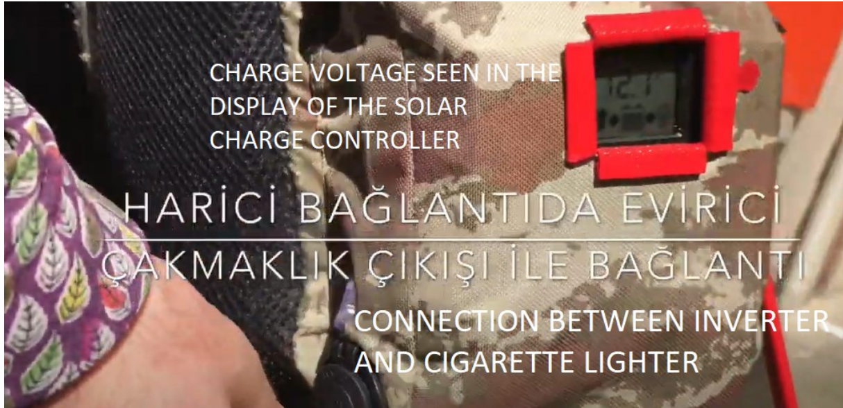
Figure 8. 12V DC output and display of the solar charge controller during charging
