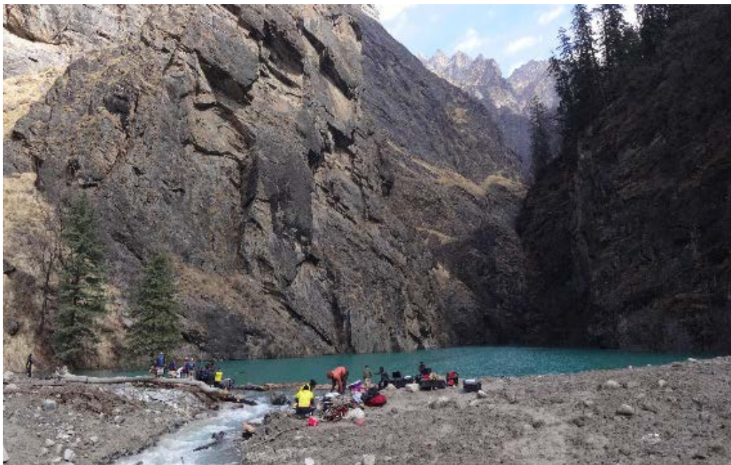
Figure 8. Personnel of ITBP and SDRF widen the channel and cleared of obstructions of logs
