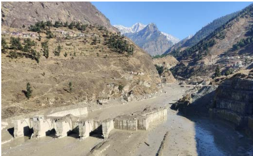
Figure 4. Severely damaged barrage of Tapoban-Vishnugad hydropower project with aggradation of river bed at Tapoban
