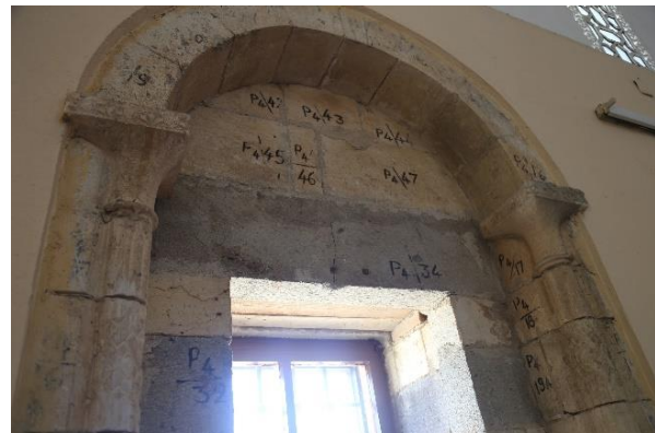
Figure 6. Cracks in the lintel above the window.
