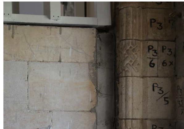
Figure 4. Stone wall joints problem in the interior.
