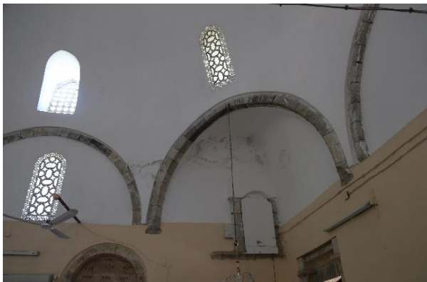
Figure 5. An example for Insulation problem.
