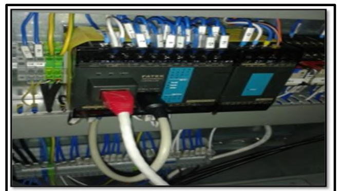
Fig. 8 PLC control unit
