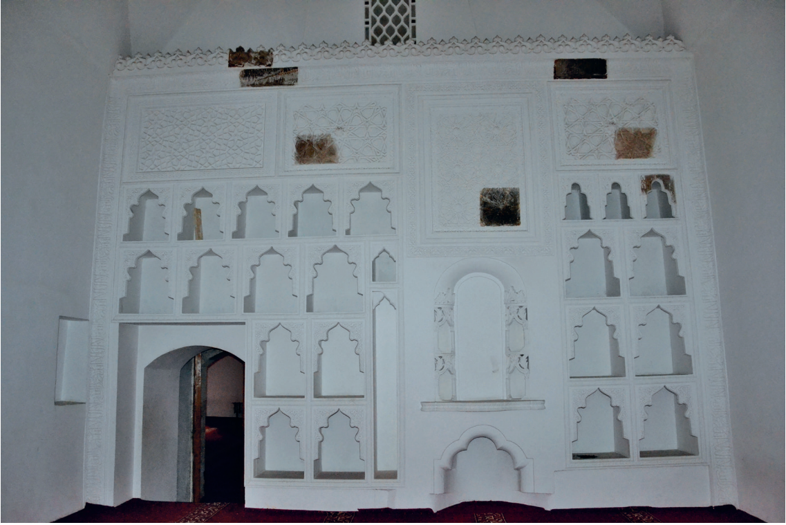
Fig. 10: The zāwiya of Bayezid Paşa (Amasya), plaster decoration in the çabâne (photograph: M. Durocher, 2017).
