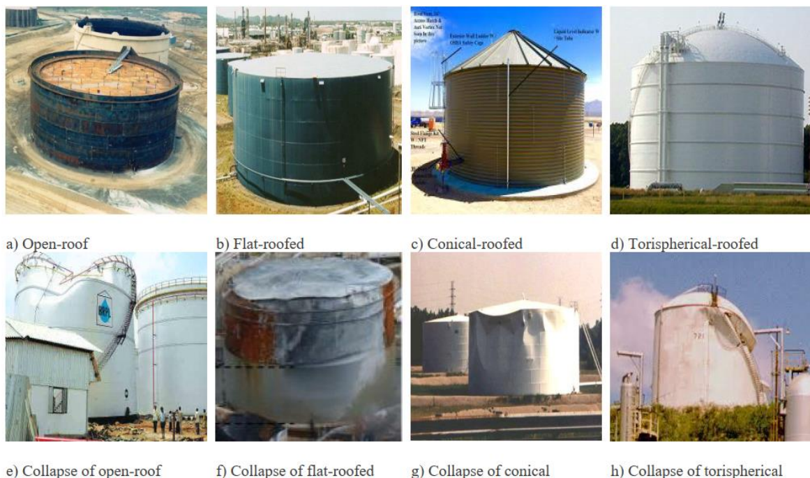
Figure 1. Types of cylindrical steel water tanks and their collapse
