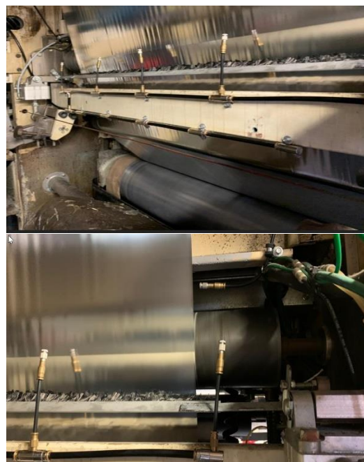
Figure 7. Dryer tunnel inlet pulverized water spray system.
