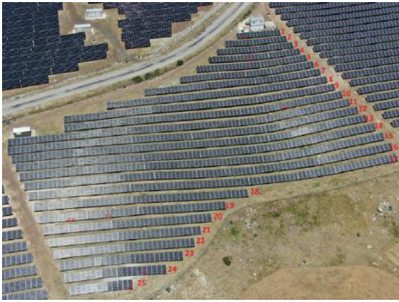
Fig. 3 2.7 MW solar power plant captured by drone
