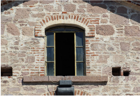
Fig. 15. Skylight Window on the Upper Level of the First Floor, Proving the Presence of an Attic (Photographed by Interior Architect Elif Türkmen)
