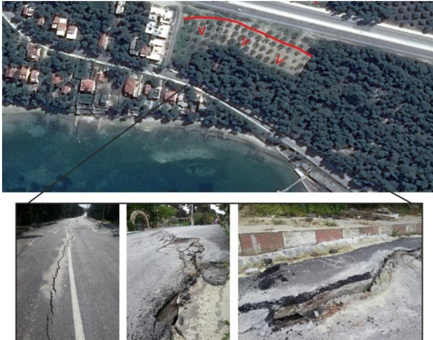
Figure 2. The view of the landslide area on the satellite image and terrestrial photographs of the landslide surface cracks.
