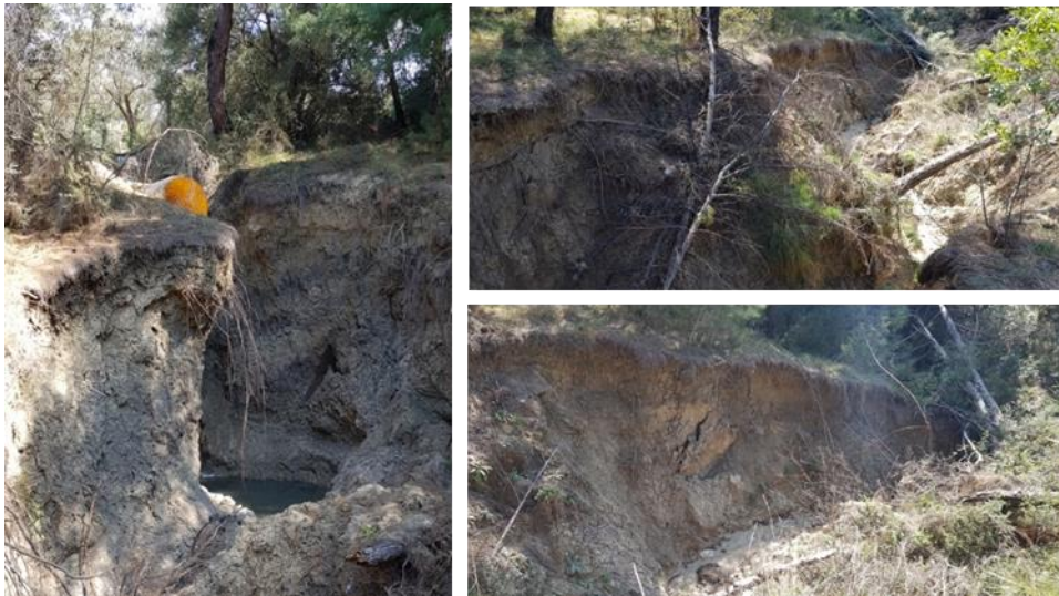
Figure 5. Soil mass change, surface deformation and its effect on vegetation caused by the drainage design on terrestrial photos.
