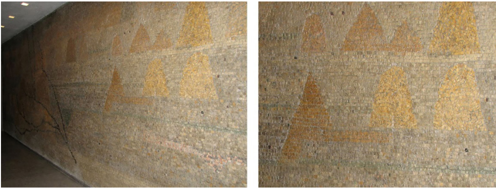
Figure 12. Detailed view of the wall mosaic with stones in conference hall foyer in the 2nd basement floor of the TMO General Directorate building. (Photographed by the author, 2008).
