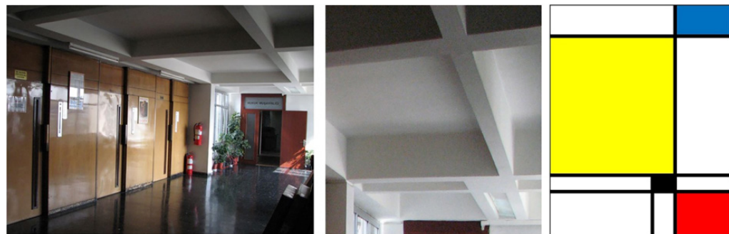
Figure 2. One of the ceilings of the service block in the TMO General Directorate building; a) general view with the wooden elevator doors and black marble floor (Photographed by the author, 2008), b) a closed view of the same ceiling (Photographed by the author, 2008), c) schematic representation of the beam plan of the same ceiling part (drawn and colored as a Mondrian painting by the author, 2022).
