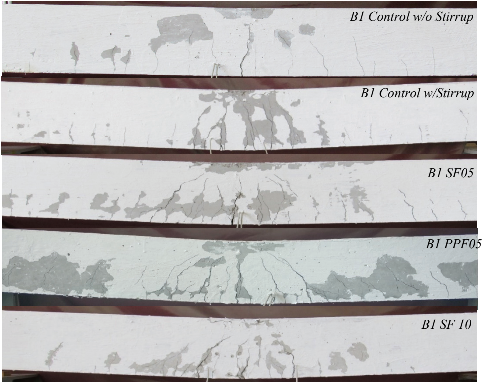
Figure 6 - Final state of crack patterns in B1 series
