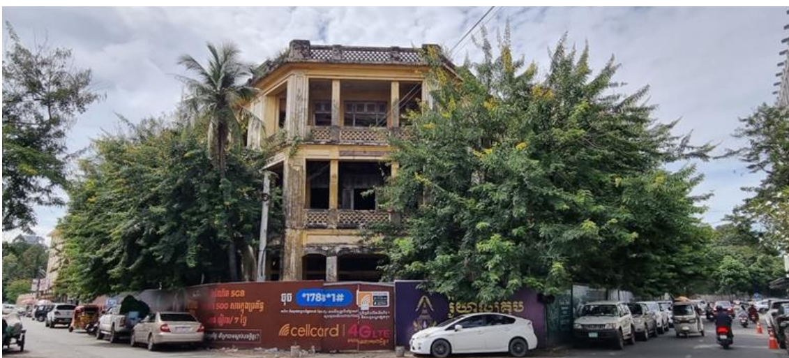
Figure 8. Dilapidated Colonial Building- Former Gendarmerie, Phnom Penh.
