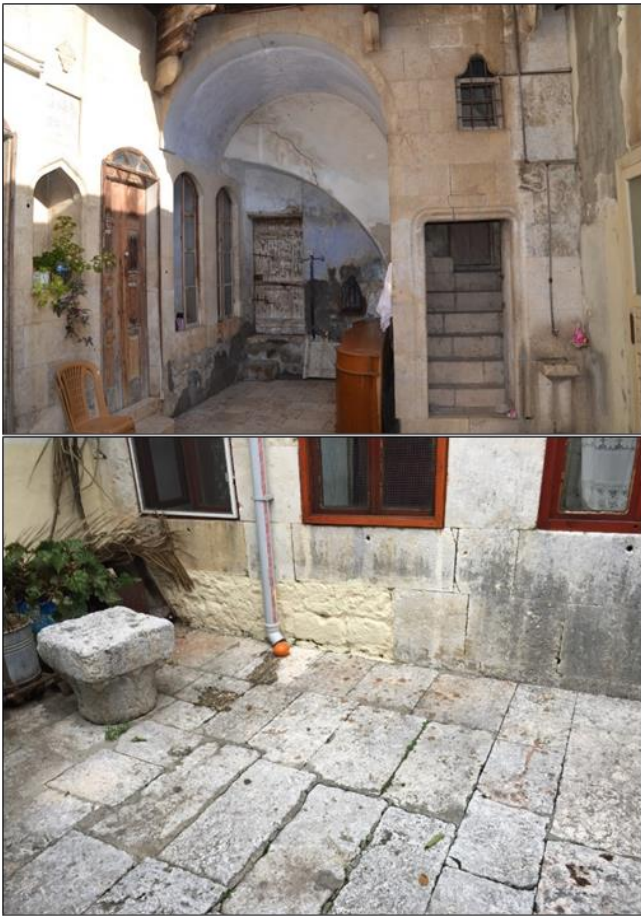
Figure 13. With respect to the comparative study on the trace on the wall and the one on the adjacent building lot no: 2060, and the statement of the inhabitant in the adjacent building in the current situation, the presence of a platform can be proposed.
