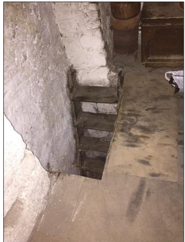
Figure 15. The ladder providing access to the upper floor in the building on the building lot no: 2060 in the 4th circumscription
