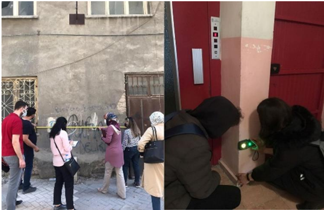
Photo 1. The damage assessment and collecting data phase of the current structure stock.
