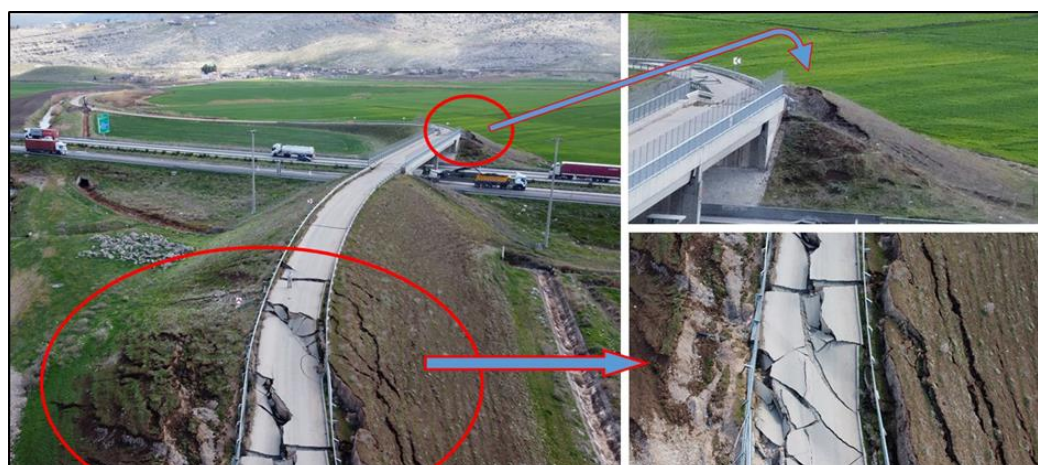
Figure 10: Gaziantep-Kahramanmaraş road Çöçelli intersection, cleavages, lateral spreading, and sinking deformations in the intersection road embankment (Figure 2).
