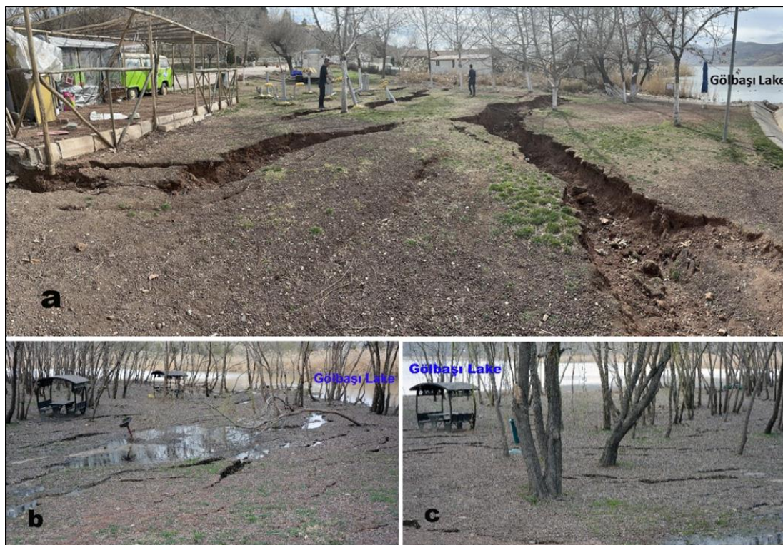
Figure 9: Lateral spreading on the shore of Gölbaşı Lake induced by the earthquake ground shaking (Figure 2).
