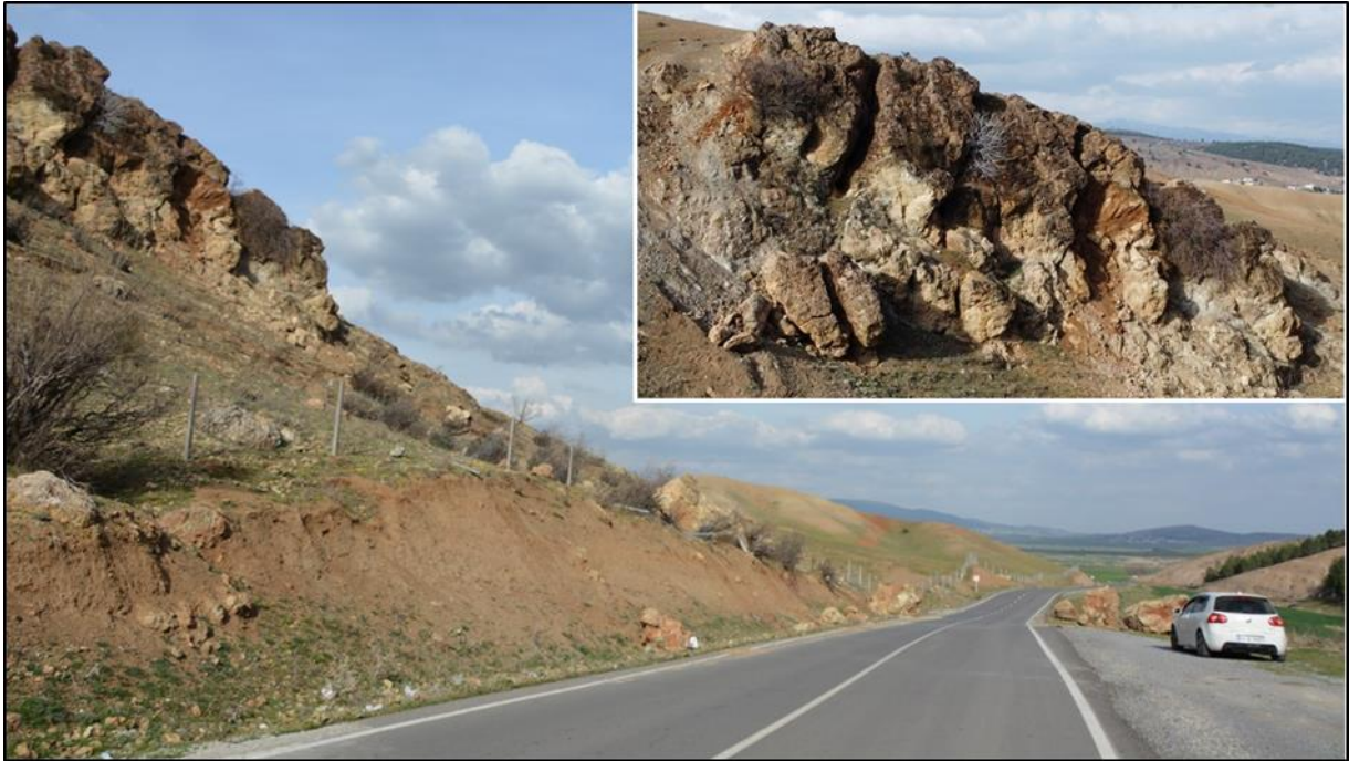
Figure 8: Kuyumcular-Kapıçam motorway, the surface rupture of February 06, 2023, Pazarcık earthquake crossing the left slope, causing large limestone blocks to break off and fall from this slope (Figure 2).
