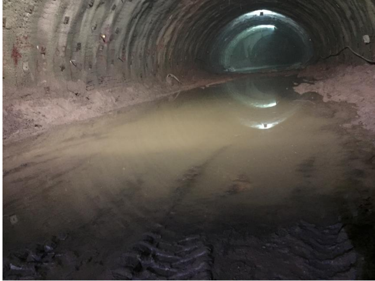
Figure 4. Water in tunnel
