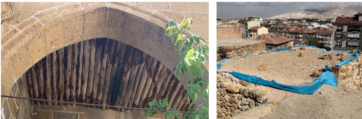
Figure 20. Round cross-section wooden beams and earthen roof forming the roof structure (author archive, 2022)
