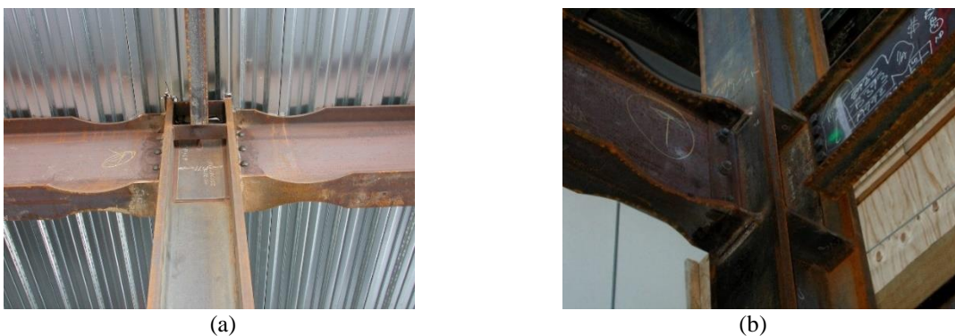
Figure 14 Column Bracing Samples: (a) Bracing at the Top Flange, (b) Bracing at the Top and Bottom Flange
