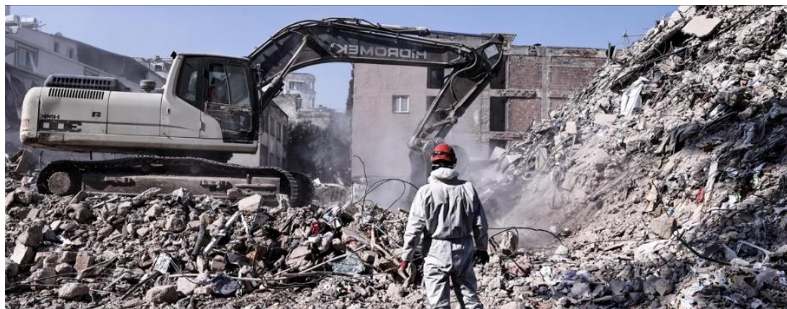
Figure 5. Destroyed area affected by the Kahramanmaraş-centered earthquake at 2023 (Palabıyık-Anatolia Agency, 2023)
