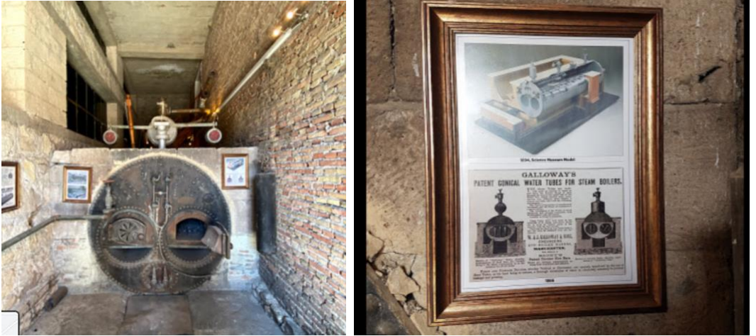
Figure 26: Güneykent Rose Oil Factory Historical Steam Boiler.
