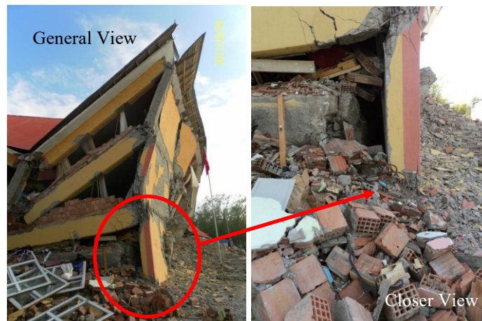
Figure 6. Failure of shear wall SW1 (E1-E2 Axis).
