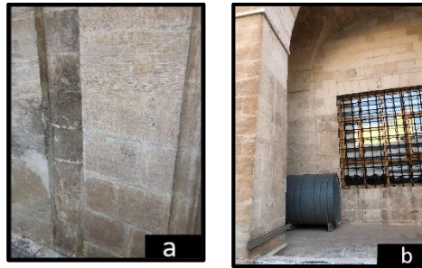
Figure 9. Anthropogenic deterioration of the Şehidiye Madrasah
