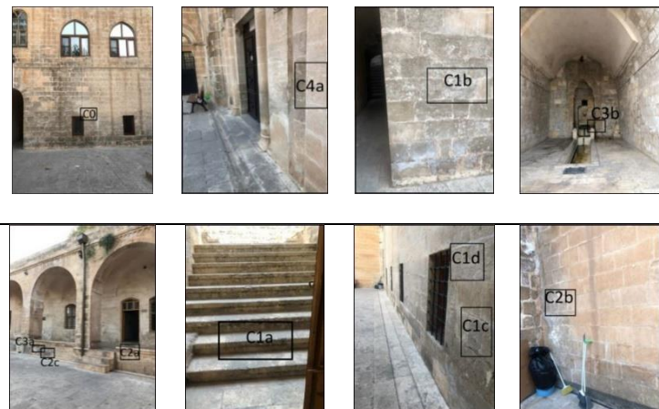
Figure 11. Demonstration of the stones selected for the use of XRF chemical method for the deterioration of Şehidiye Madrasah on the façade
