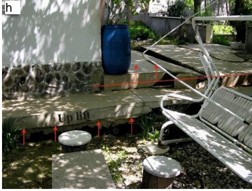
Figure 5. a) Separations in adjacent buildings and incorrect infrastructure, b) vertical displacement of garage entrance from the road level, c-d) building tilted backward by landslide, e-h) deformations of the road, garden walls and structures.
