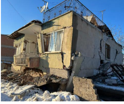
Figure 28. Corner collapses due to vertical cracks in Akçadağ
