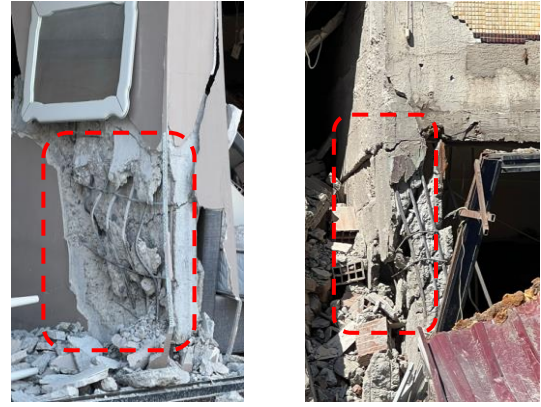
Figure 11. The observed damages in the old buildings in the city center, caused by the insufficiency in stirrups and the use of non-deformed steel bars
