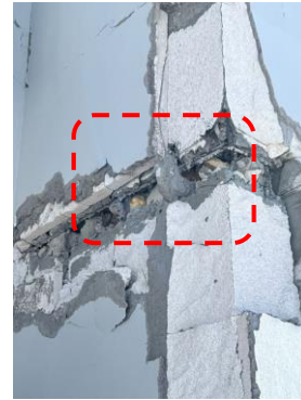
Figure 16. Foreign materials in concrete
