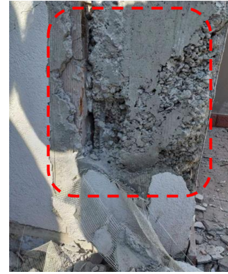
Figure 15. Insufficient concrete cover, concrete settlement problems and segregation
