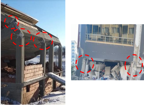
Figure 18. Stability problem due to weak column-strong beam situation
