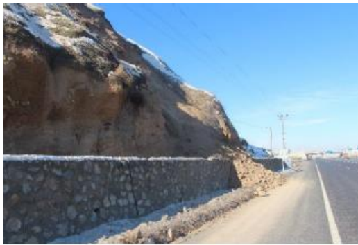
Figure 32. Retaining wall failures and flow of backfill material
