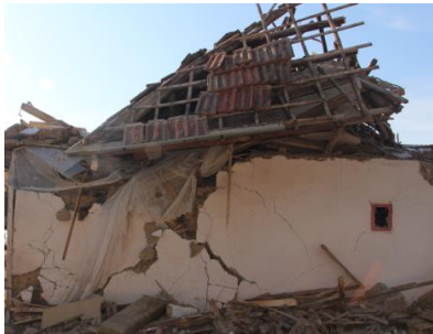
Figure 25. Collapsed structures in the rural areas
