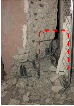
Figure 14. Rupture in stirrup and buckling of longitudinal reinforcement
