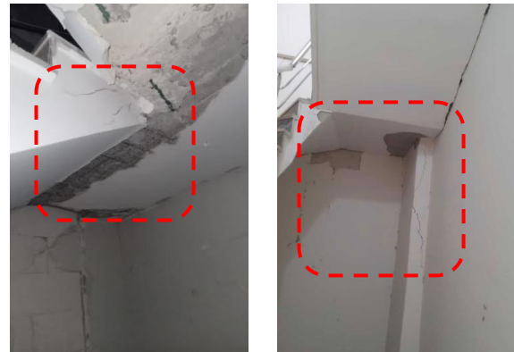
Figure 17. Damages in staircase
