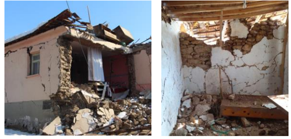
Figure 26. Wall damages in Gündüzbey and Akçadağ
