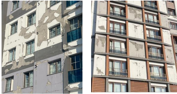
Figure 21. Cracks and plaster spills observed on the exterior of the buildings
