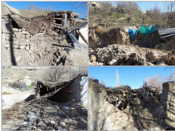
Figure 8. Example of partial collapse damage of heavy earthen roofs
