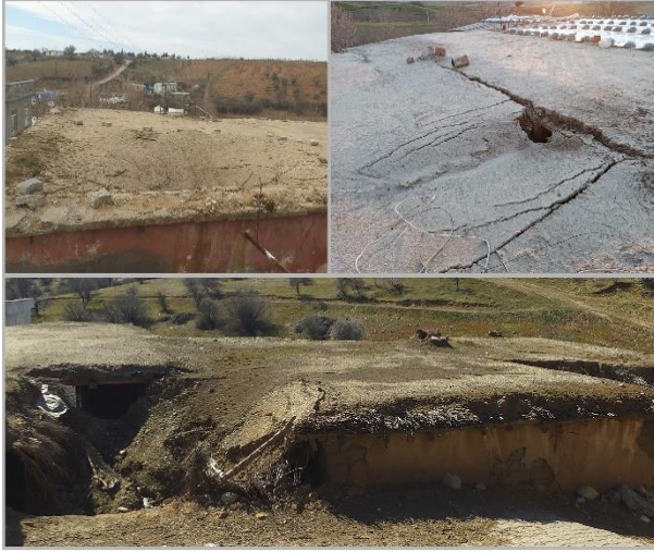
Figure 12. Example of the structural damage on flat earthen roofs
