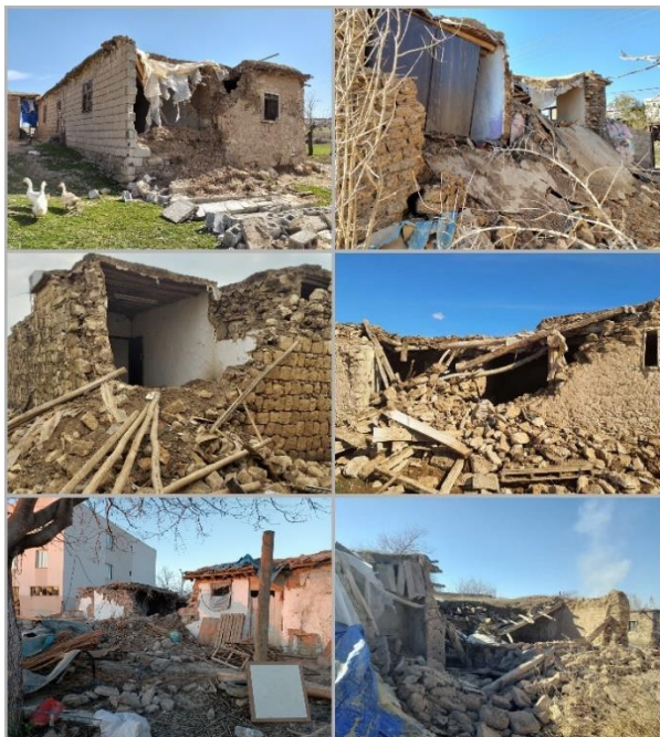
Figure 9. Load-bearing wall damages due to partial collapse of heavy earthen roofs
