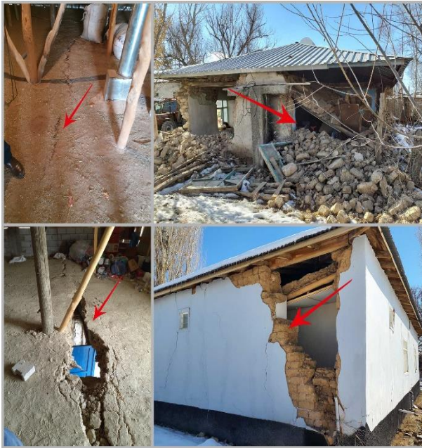
Figure 13. Examples of damage to earthen roofs with wooden roof rafters
