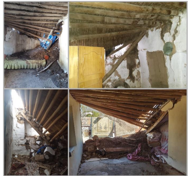
Figure 10. Damages due to insufficient support of wooden beams on heavy earthen roofs
