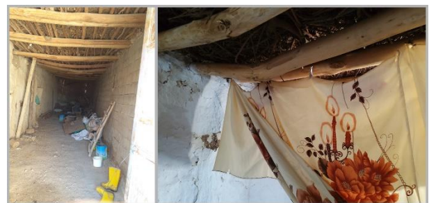
Figure 11. Examples of wooden beams forced to collapse
