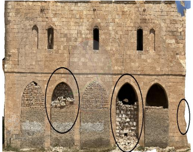
Figure 8. The deformed walls
