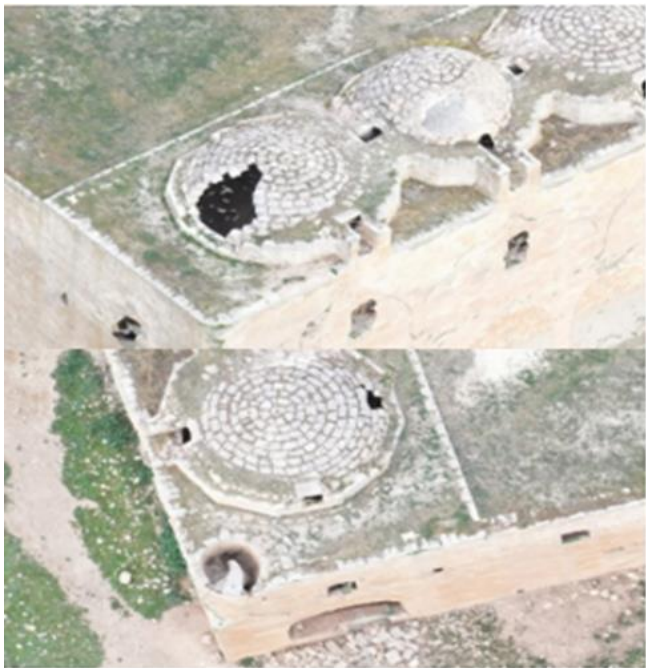
Figure 7. The deformed dome.
