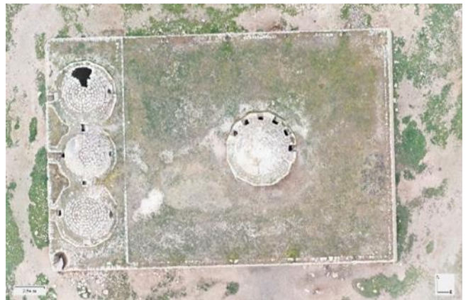
Figure 9. Soil accumulation and grass on the roof of the church
