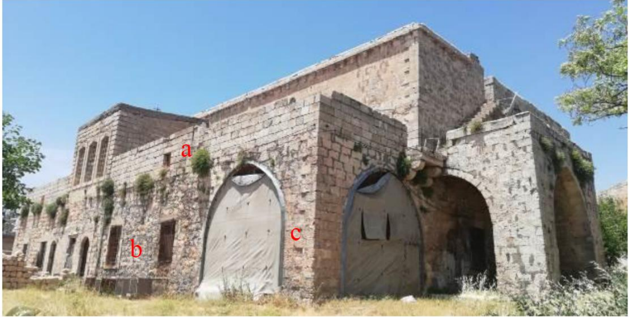
a. Plant formation b. Use of cement c. Loss of surface
