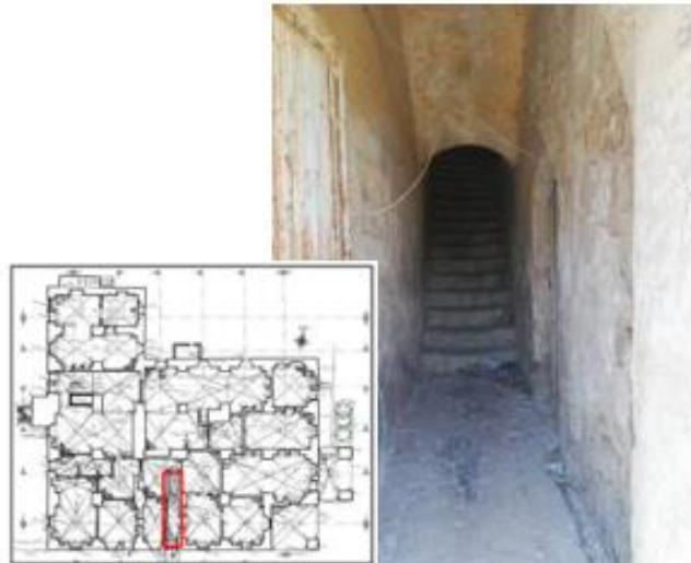
Figure 16. Tear and colour change on the stairs (Karataş,2
