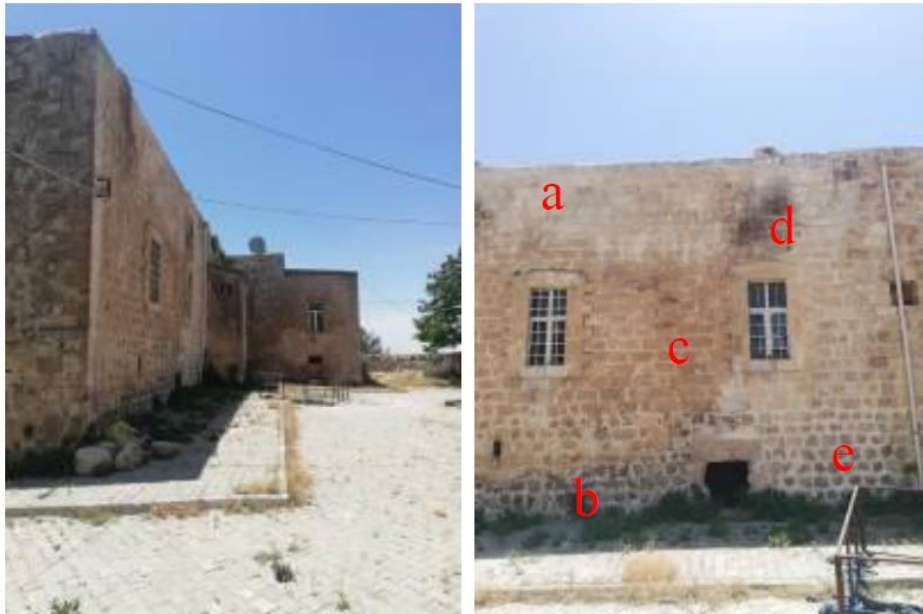
a. Efflorescence b. Plant formation c. Colour change d. Surface contamination e. Use of cement
