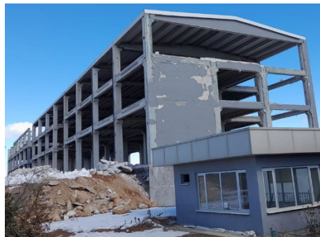
Şekil 6: Deprem hasarı almış 3 katlı betonarme prefabrik yapı Figure 6: 3-storey reinforced concrete prefabricated building damaged by earthquake
