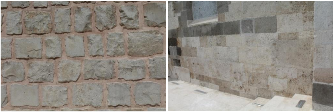
Figure 3. Facade cleaning carried out on the mosque's east facade and north courtyard facade rough masonry stones
