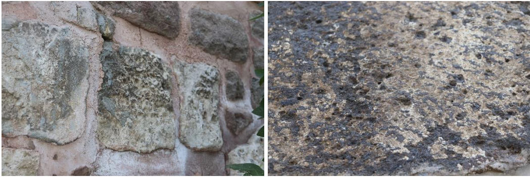
Figure 16. Biological (Moss, Lichen etc.) formations on stone surfaces
