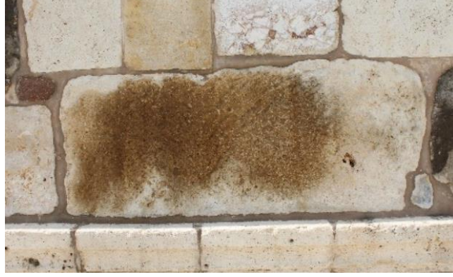
Figure 15. Abrasion on stone surface due to chemical effects
