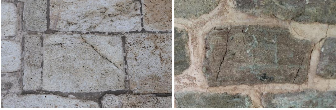
Figure 12. Crack - fracture formations on the stone surface
