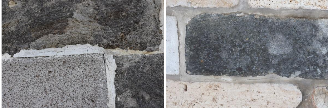
Figure 13. Crack formation in joints due to thermal expansion
