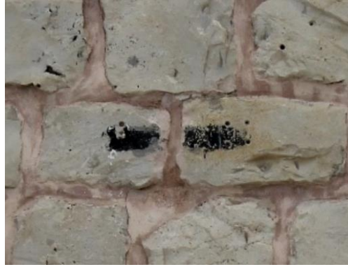
Figure 18. Pollution caused by paint and similar marking tools
