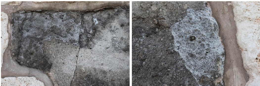
Figure 14. Defects caused by air pollution and exhaust gases
