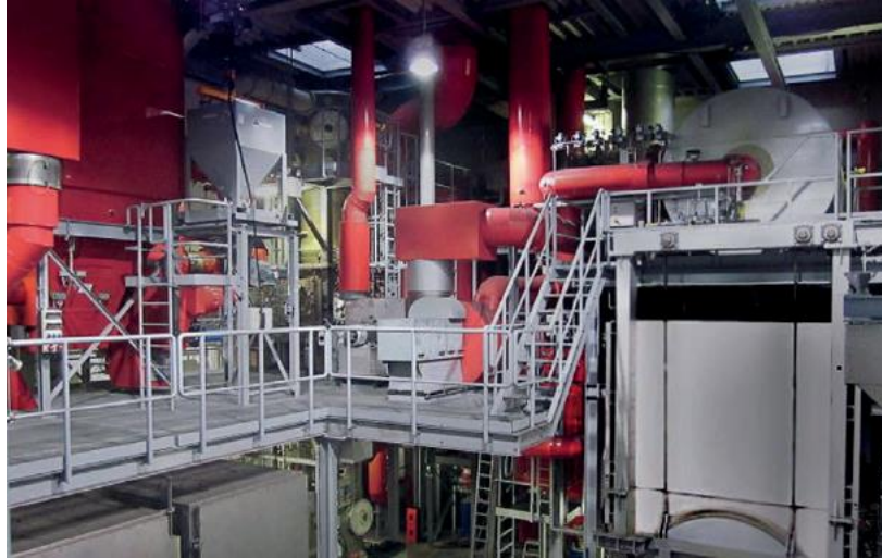
Figure 4: A limestone flue gas desulfurization plant [5].
