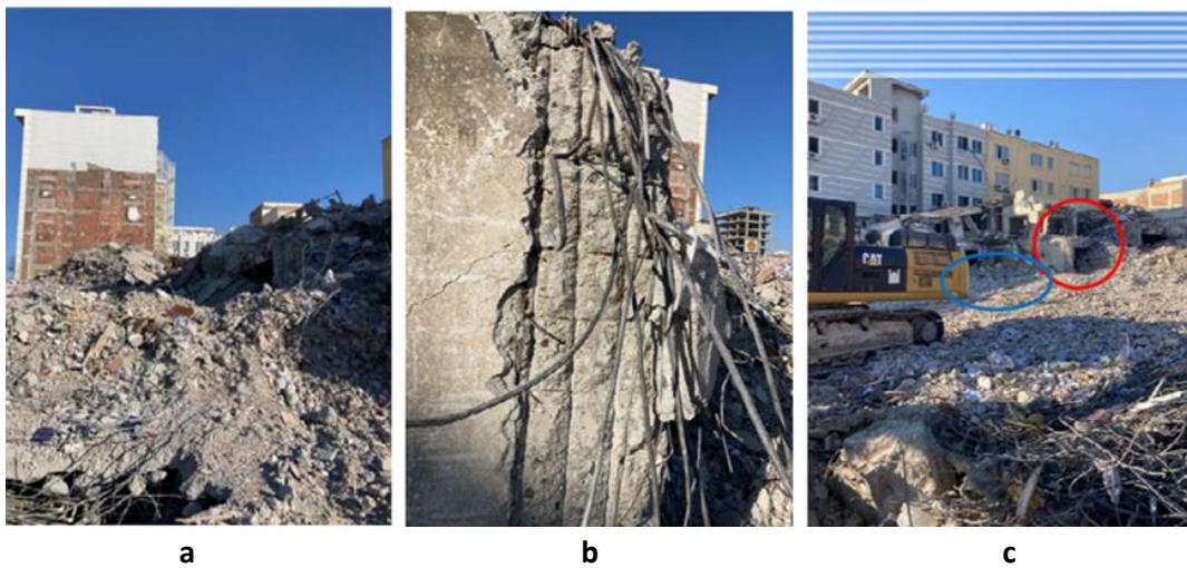
Figure 4. a-b. Overall view from the debris field with the intact 7-story building in the background (EMU, 2023). c. Columns from the undamaged part of the hotel (EMU, 2023)
