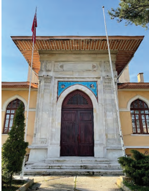
G. 4: Edirne Union and Progress Club Building, Crown Door View, (A. Balci, 2022)
