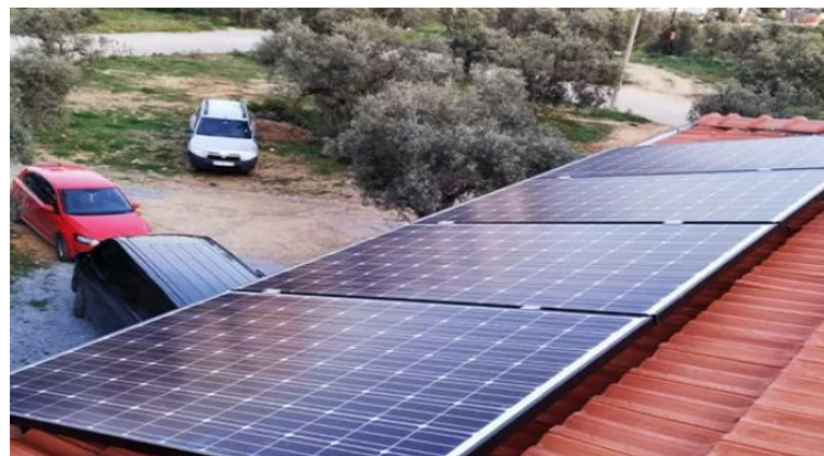
Figure 12. Excel PV-T Hybrid solar panels (Solimpeks, 2023).
