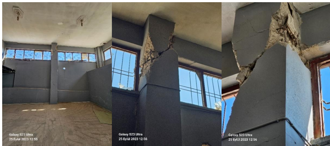
Figure 8. Short colon effect damages – Malatya (Karataş, 2023)
