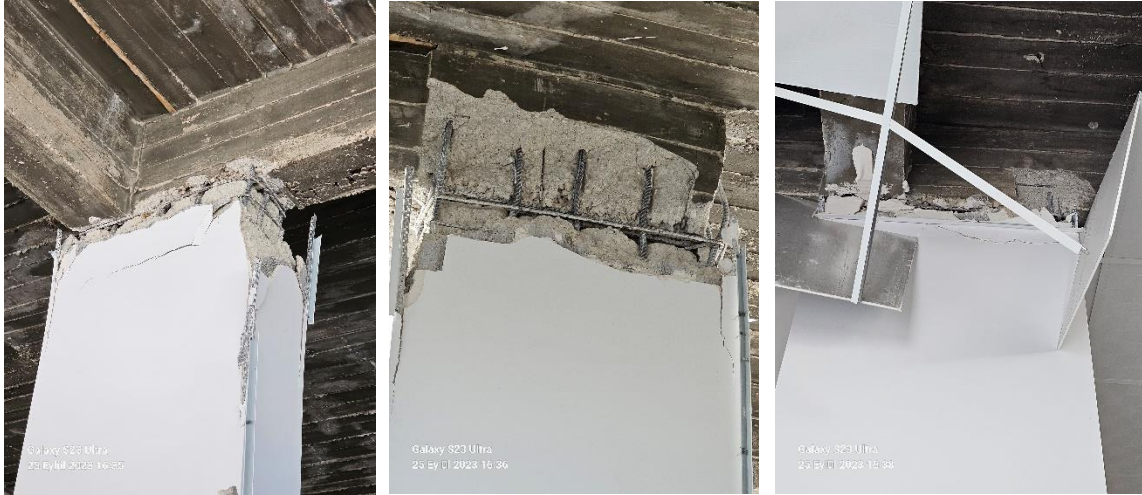
Figure 9. Weak column and strong beam damage - Malatya (Karataş, 2023)
