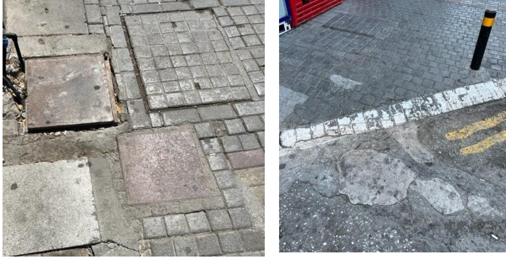
Figure 6. Poor Maintenance Facilities Pose Danger During the Usage of Pedestrian Routes (Güvenbaş, 2023)
