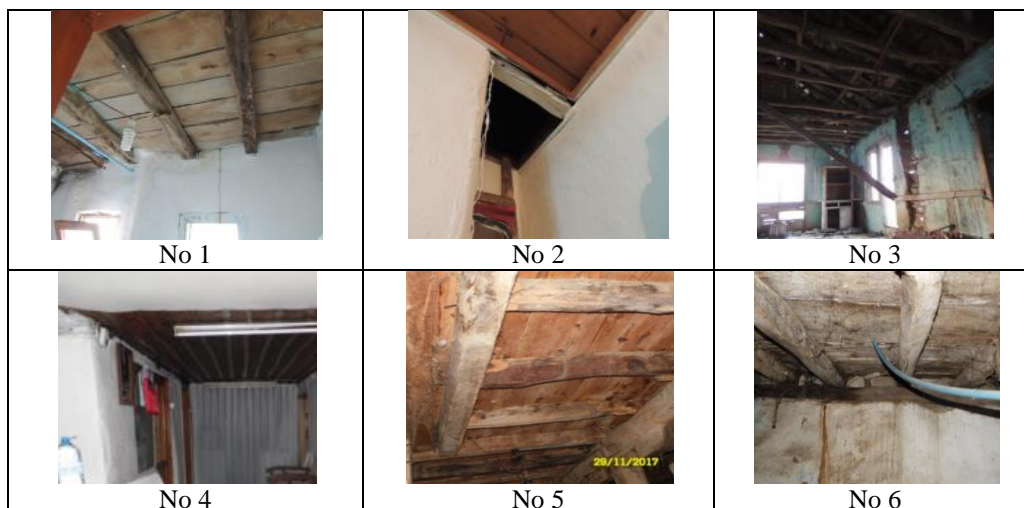
Figure 11. Ceiling Images of Houses No. 1, 2, 3, 4, 5, and 6
