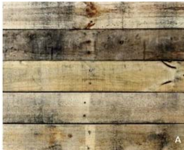
Figure 2. Mold fungi (Is It Really Mold or Just Staining? CONNER Industries, 2024).
