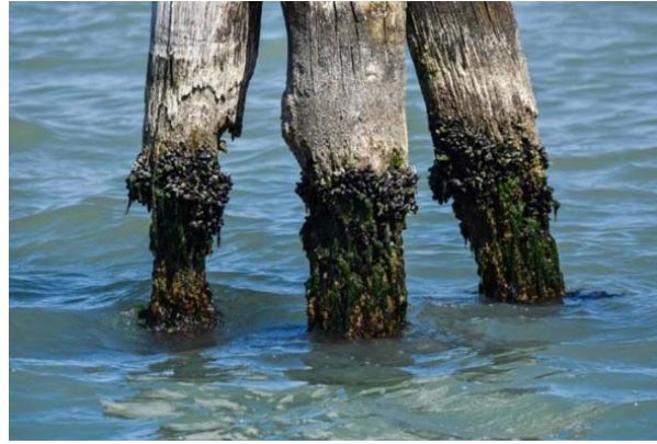
Figure 12. Damage on wood in marine (Wooden bricole, wooden mooring poles in the water, Venice, Italy, 2019 Free Photo, 2024).
