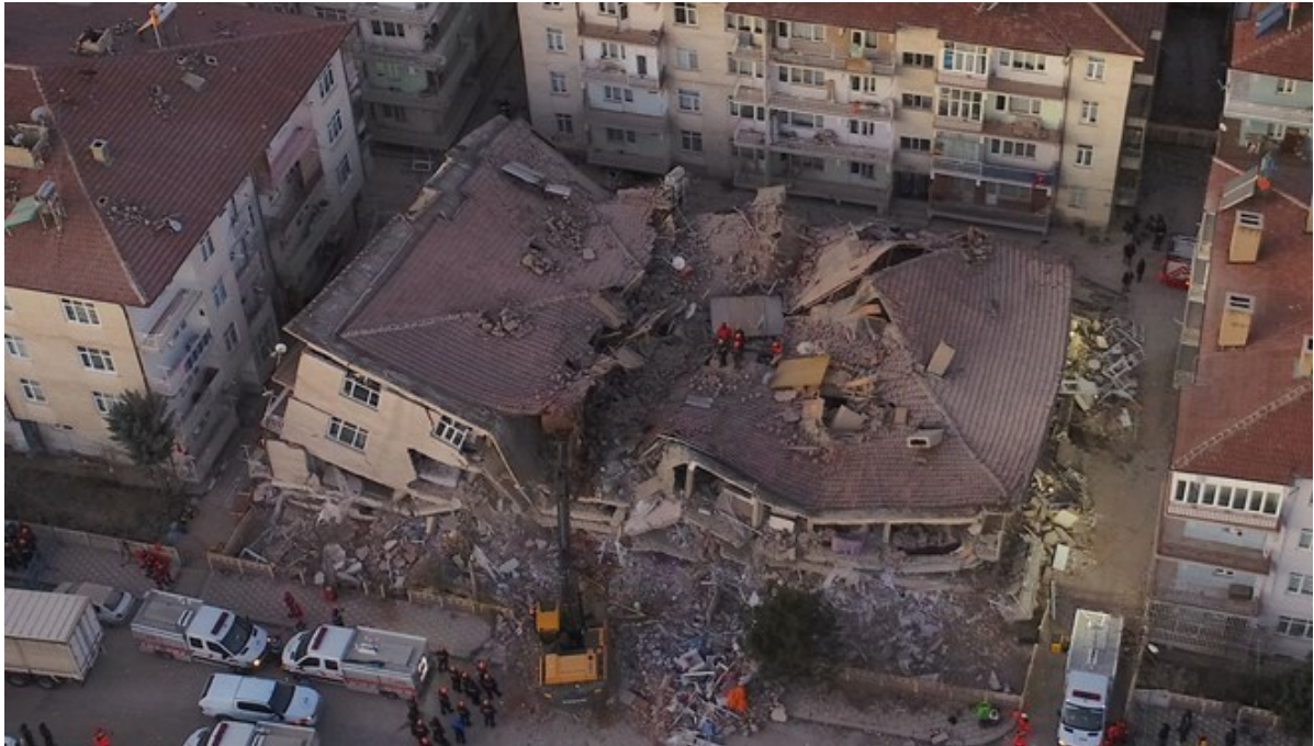
Figure 6: 14 people died in Dilek apartment building. Source URL 1.
