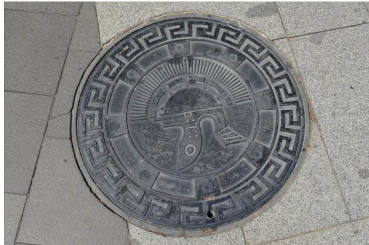
Figure 7. The drain covers used in the complex.
