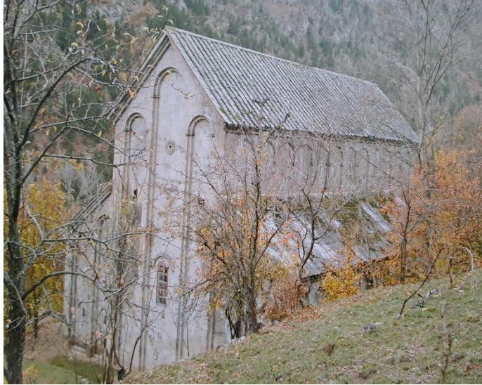
Figure 12: Church of St. John the Baptist of the Parhal Monastery, north-east (Kadiroğlu ve İşler, 2010: fig.52)
