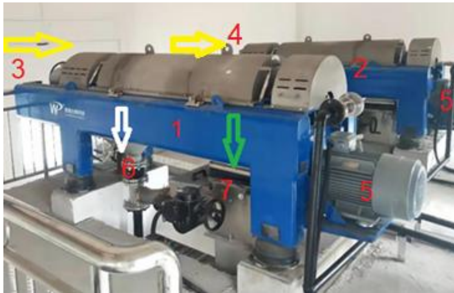
Figure 1. The decanter unit considered in this study 1&2 Decanter units (main and spare one), 3&4 Sludge feeding, 5 Decanter electric motor 6-Separated liquid output 7-Separated solid output
