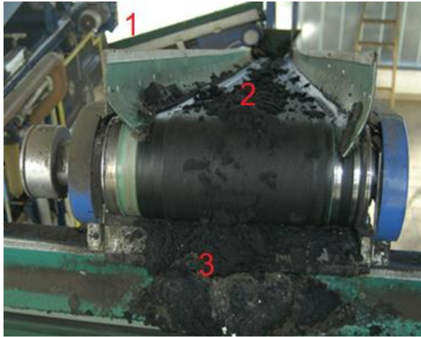
Figure 2. Sample sludge conveyor unit 1-Conveyor belt feeding from decanter, 2-Conveyor belt sludge transfer, 3-Sludge sampling point
