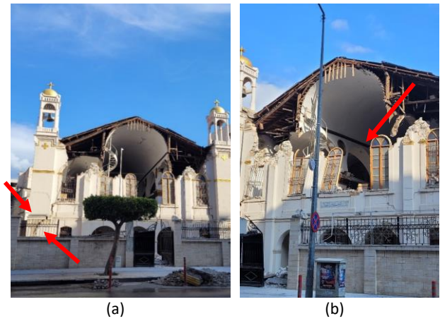
Figure 19. St. Nicholas Orthodox Church in Iskenderun, (a, b) Observed combined in-plane and out-of-plane mechanisms in the St. Nicholas Orthodox Church after the earthquake.
