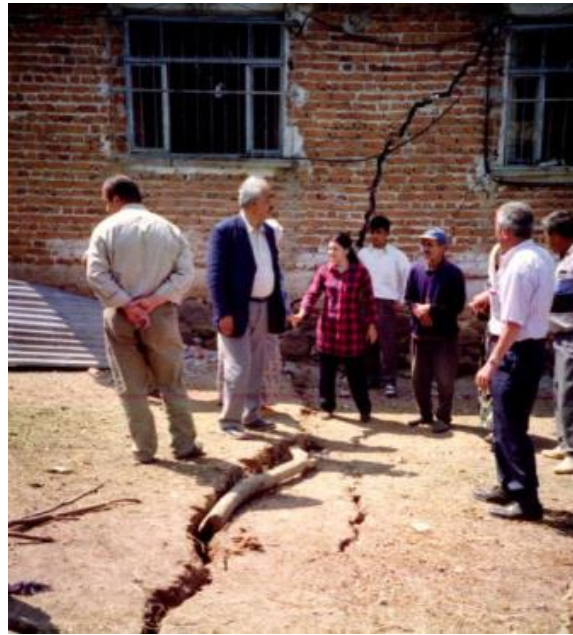
Figure 1. Damages Resulted From Blasting-Induced Ground Displacement (Köksal & Karaca, 2018)
